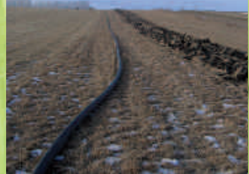
Glass fiber-reinforced polyethylene pipe is installed quickly with minimal disruption to the environment.
