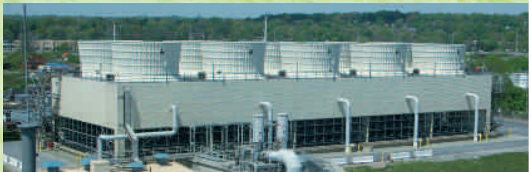
One of Bedford Reinforced Plastics' largest applications is cooling towers for power plants.
