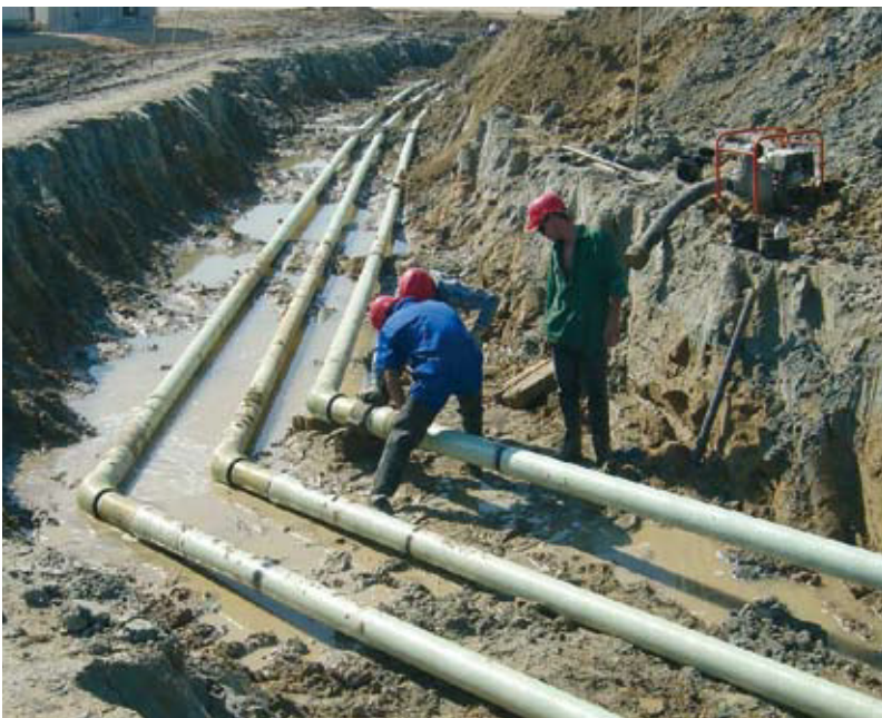
Infrastructure projects in Asia Pacific include municipal pipe in China, India and Australia.
