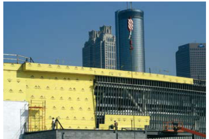
Owens Corning worked with Georgia-Pacific to develop and introduce a non-woven facer for its DensGlass Gold® exterior sheathing product.
